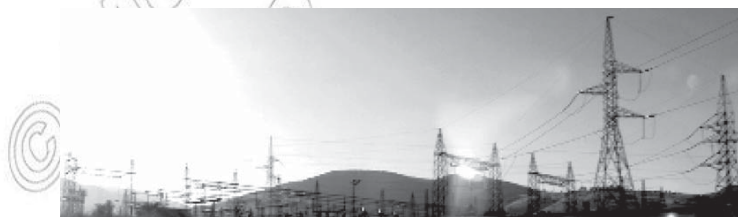
High voltage power lines and pylons
